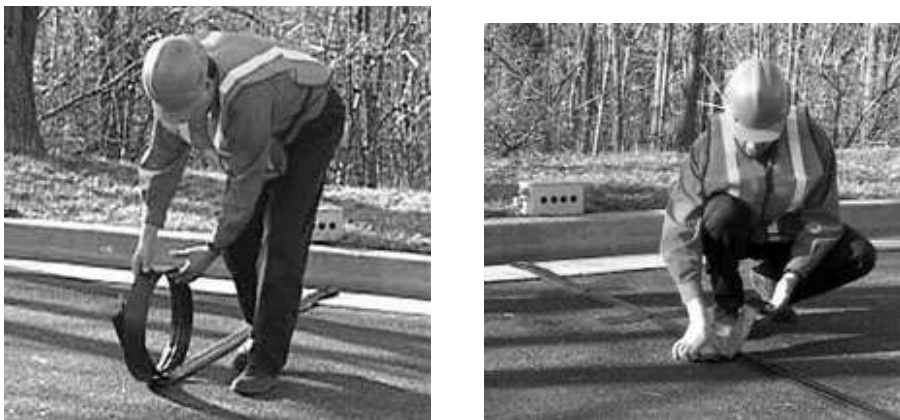
Figure 2.4: The installation of a mobile pneumatic tube traffic detector. The tube is fixed on the road surface and connected to a registration unit at the roadside. (Photo courtesy of PET Corp)
