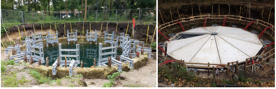
Figure 8.3: Construction of the STESS. Left: installation of the last heat buffer. Right: STESS almost completely sealed.
