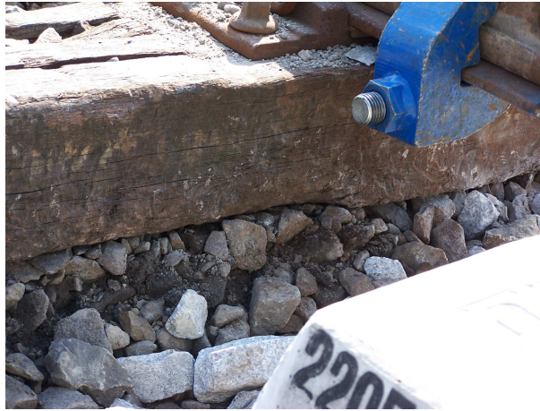
Figure 1.2: Severely worn ballast stones under an old sleeper. Compared with the new ballast stones nearby with sharp edges, the worn ballast stones have become rounded in shape and covered by dust. This problem is called the "foul" of the ballast, meaning that the ballast stones have been crushed, provide less drainage, move less, and have less elasticity, leading to a reduction in their friction dissipation.
