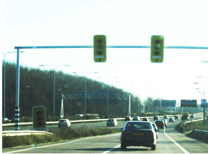
Figure 1.3: On-ramp metering installation.
