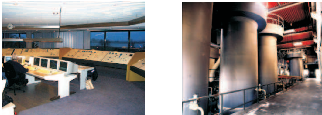
Figure 16: The control center of the Amsterdam Water Supply plant (left) and the softening reactors (right).
