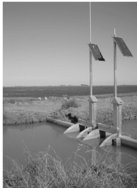
Figure 4: Overshoot gates on Coleambally Channel Number 6 (Source: Rubicon Systems Australia Pty. Ltd)
