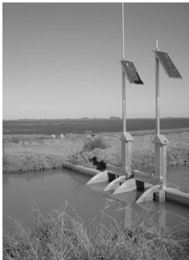
Figure 4: Overshoot gates on Coleambally Channel Number 6 (Source: Rubicon Systems Australia Pty. Ltd)
