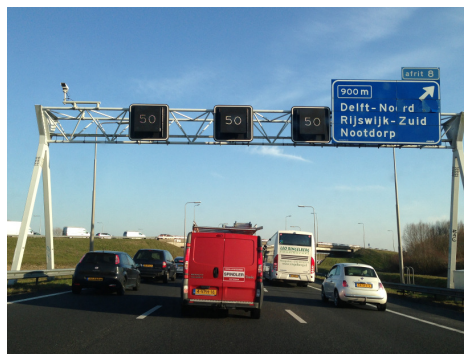
Fig. 1. VSL implementation on A13. Delft, The Netherlands.
