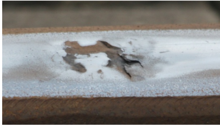
(a) Picture of the defect
