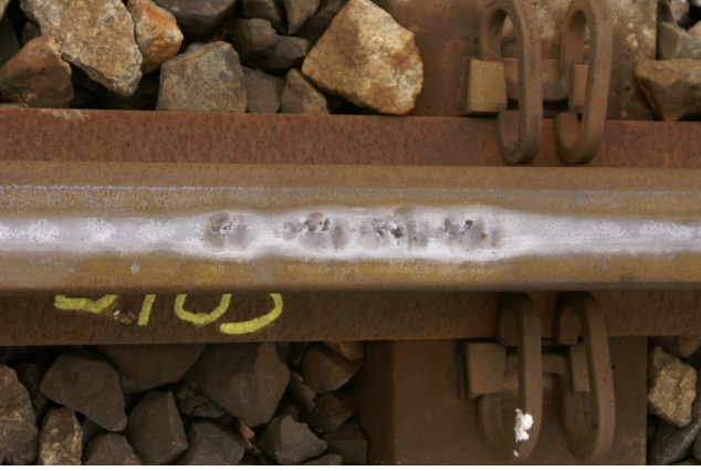
Fig. 1. Example of severe squats on a rail
